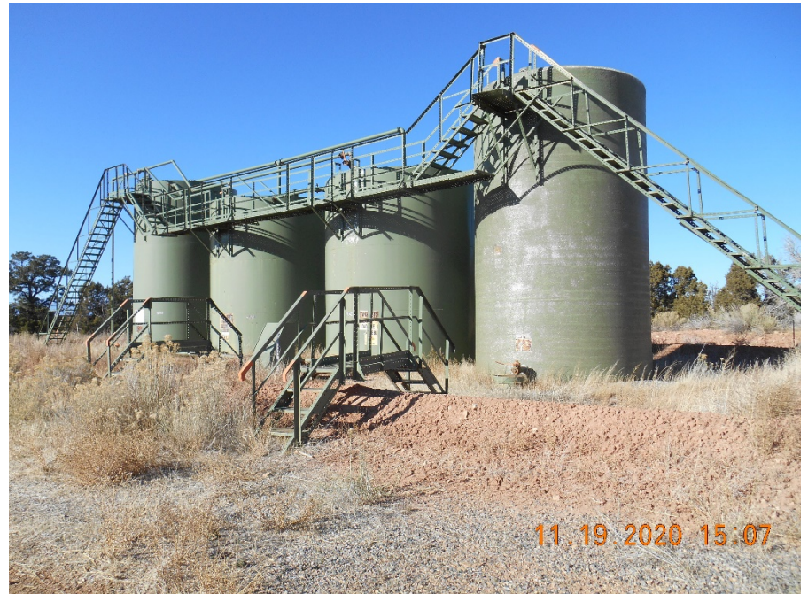
Tank Battery with earth berms.
