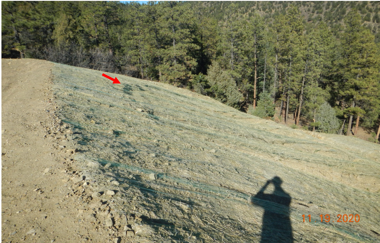
Photo 4. Facing northeast. The arrow points to an outline in the embankment which appears soil has moved. This area needs to be monitored for stabilization.
