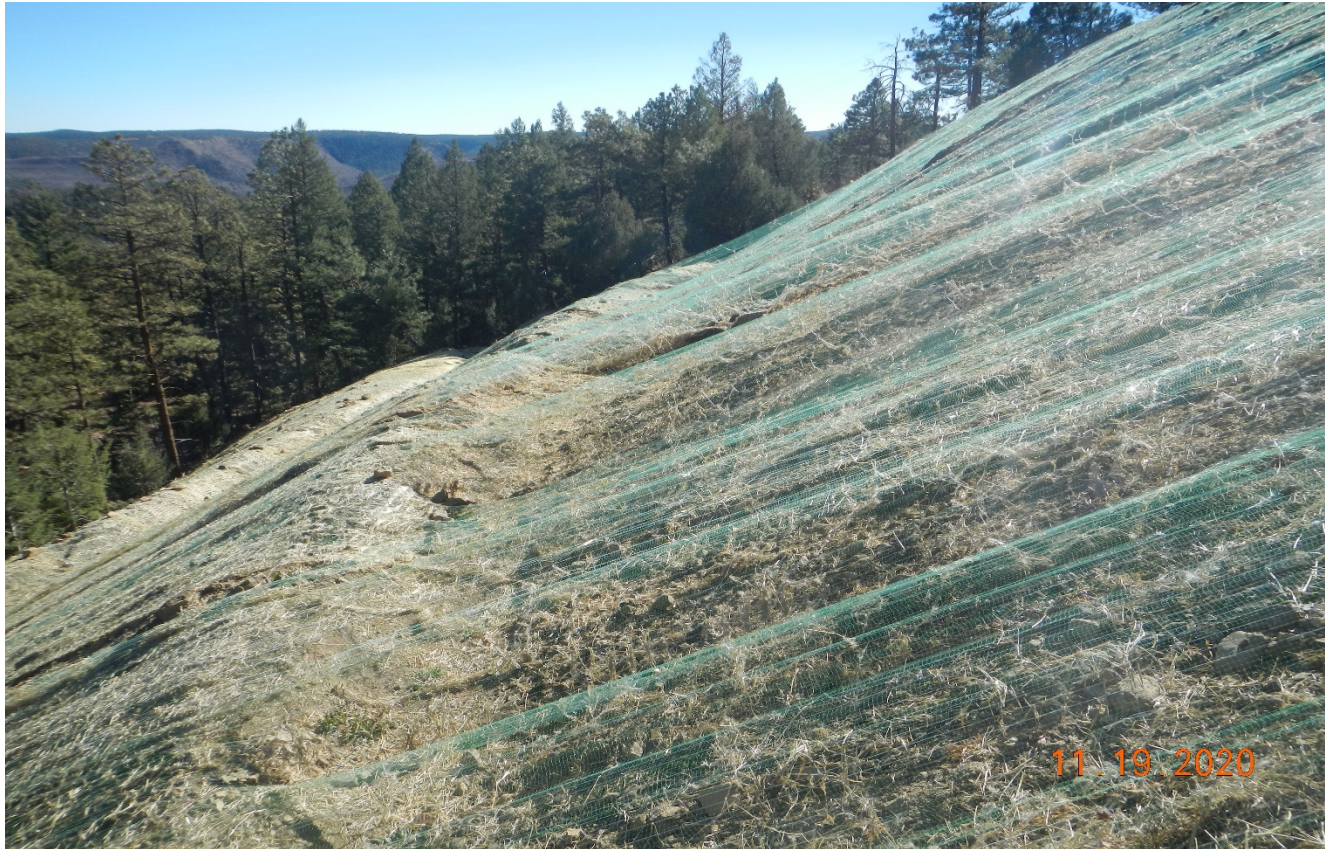
Photo 3. The straw blanket is stretched out likely due to soil movement.
