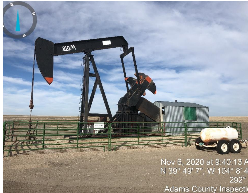
Photo #1 Pump Jack.
