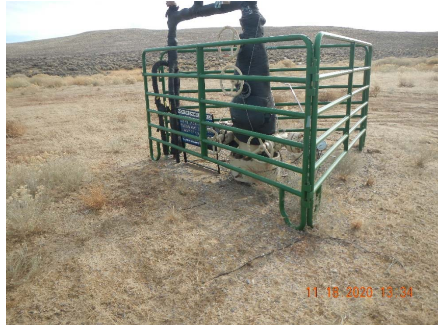
Photo 2. No bradenhead access apparent.
