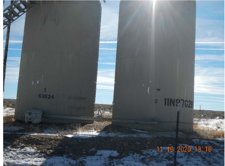
Photo 3. Missing tank labels.
