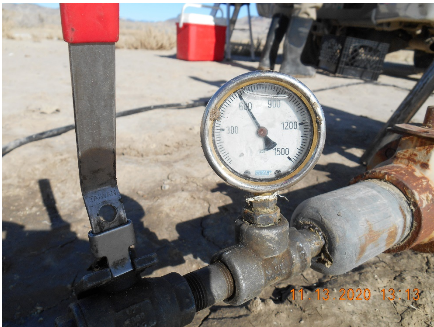
Gauge at start of test
