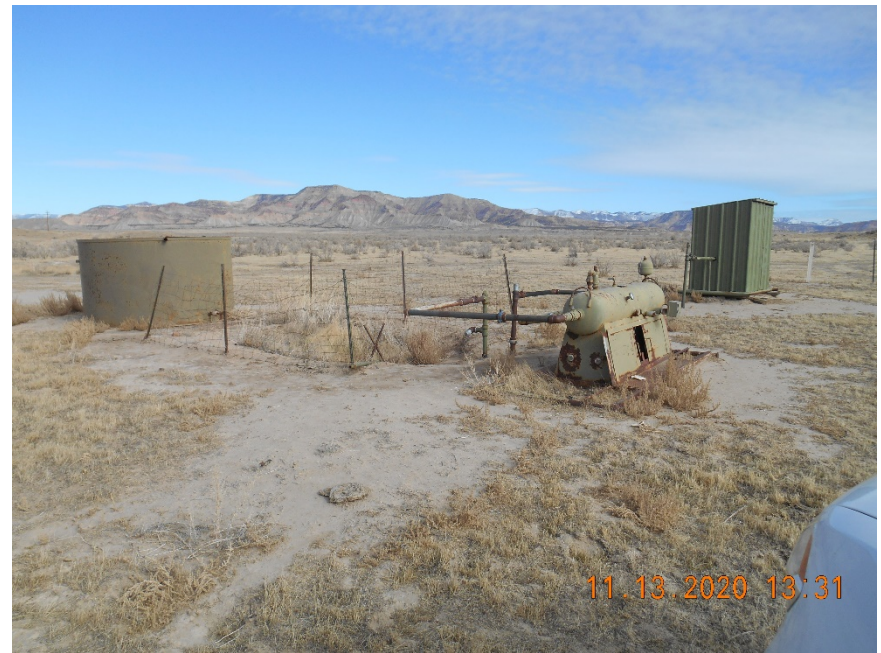
Separator , meter housing , tank and blowdown pit.
