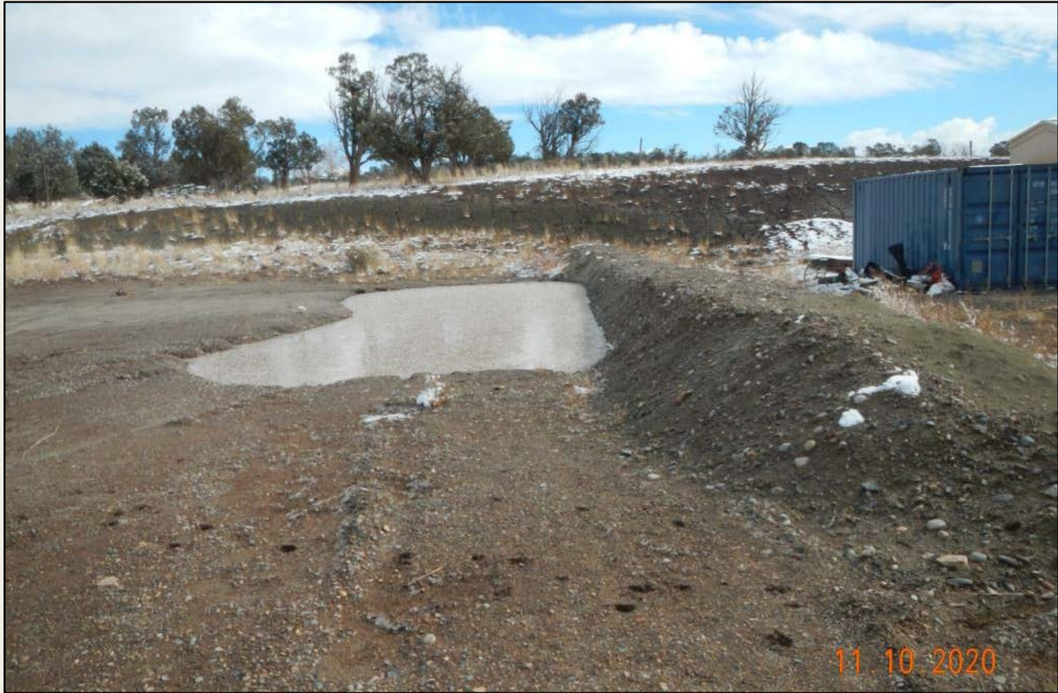
Photo 3. View of area in the southern project area where berm and silt trap installed.
