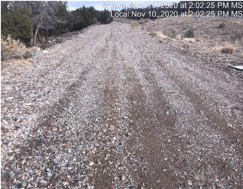
Photo #2236 Tracking occurring from location to access road.
