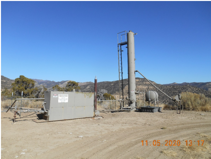
Separator and Dehydrator
