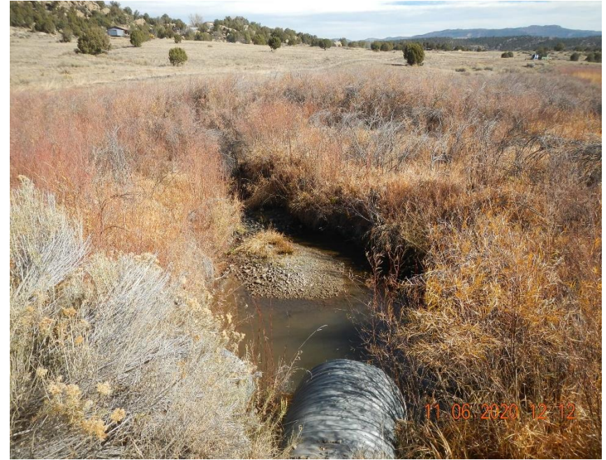
Unnamed drainage impacted by fluids from Spill/Release Point ID #478491.
