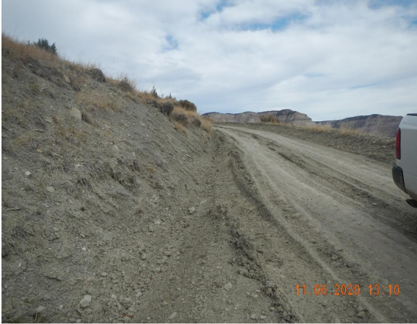
Vehicle tracks running into ditch.
