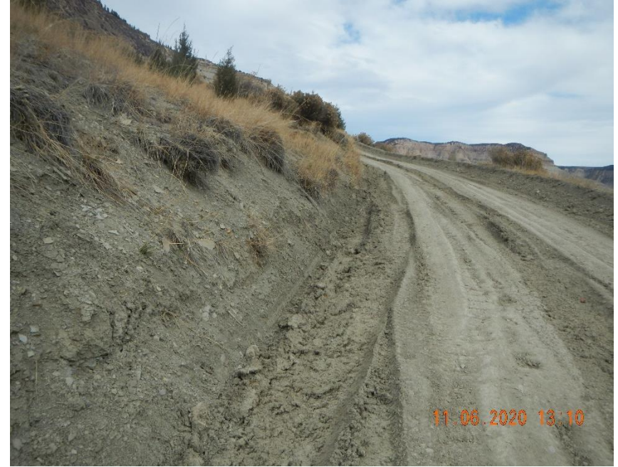
Vehicle tracks running into ditch.
