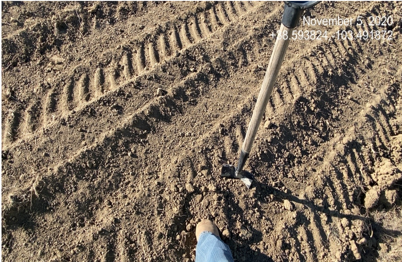
Photo 4. The topsoil pile has been tracked but is not sufficient to stabilize and maintain the topsoil pile. The topsoil is susceptible to erosion.
