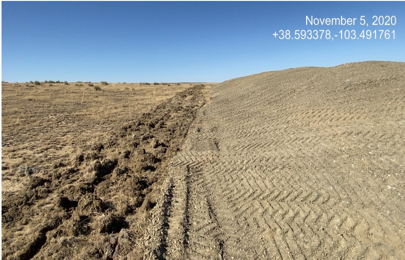
Photo 6. Soil roughening has occurred around the location.
