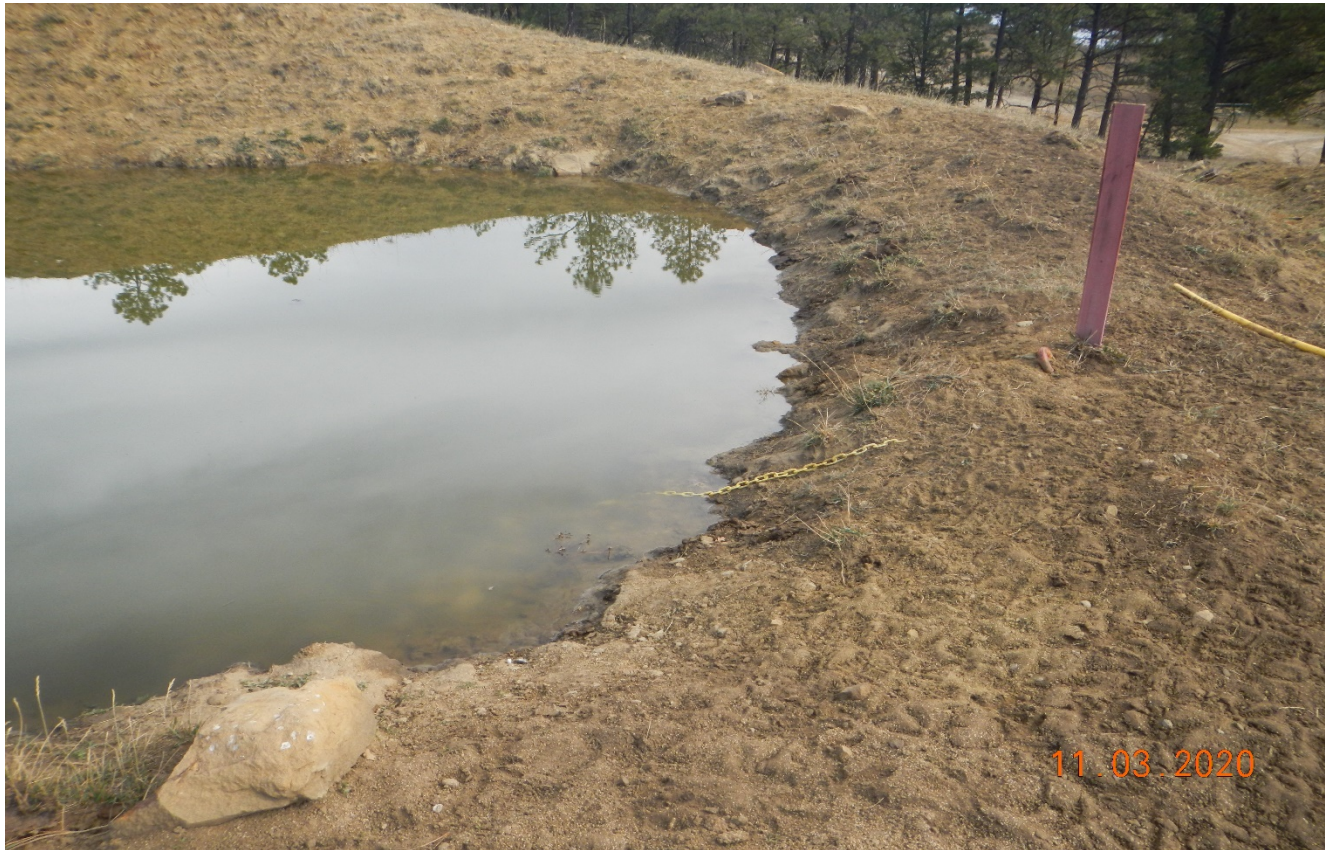
Photo 3. Water level in pit is above 2 ft. freeboard.
