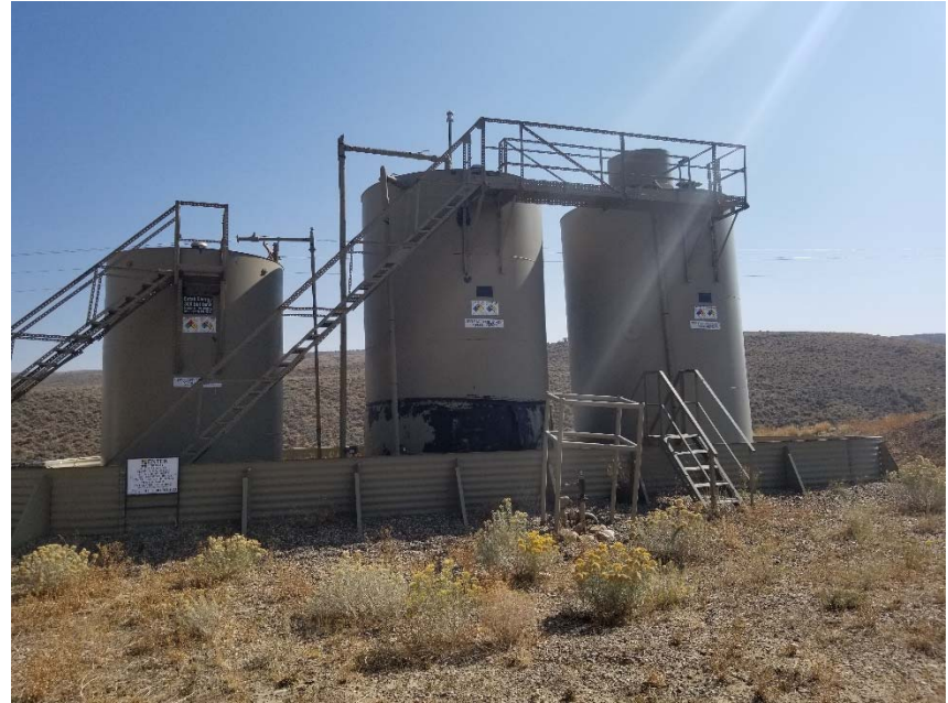
Photo 4. Crude tanks with berm.
