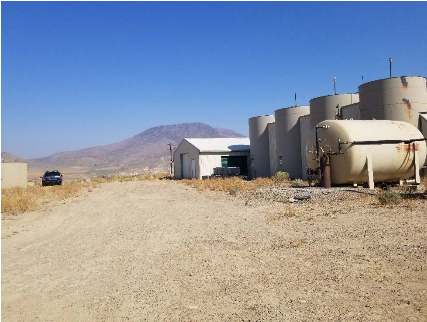
Photo 3. Produced water tanks with no berm.
