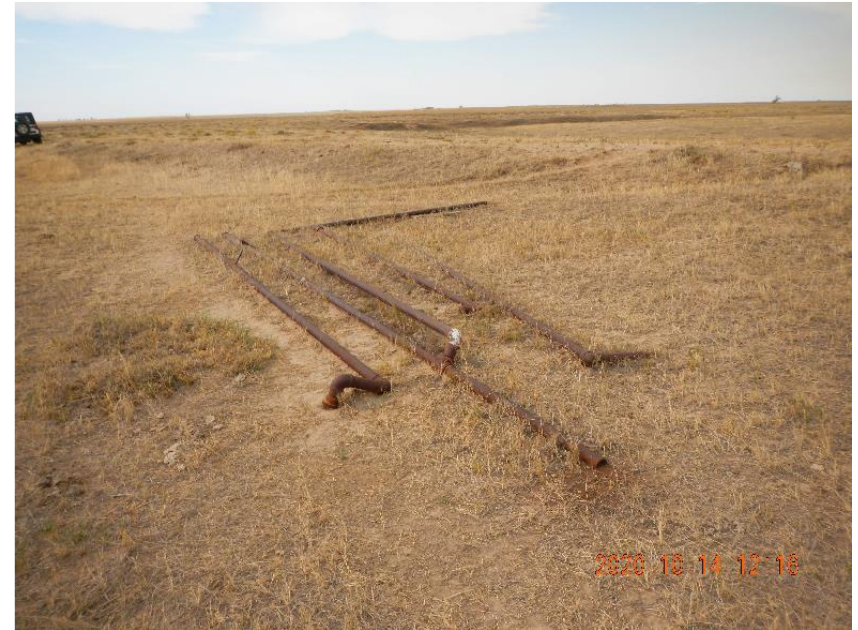
Photo 6: Disconnected pipe at well location.
