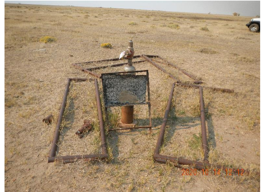
Photo 4: Additional view well and downed steel pipe barrier.
