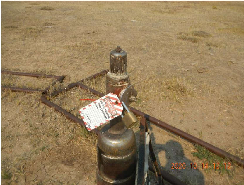
Photo 5: Locked valve and bull plug on casing string.
