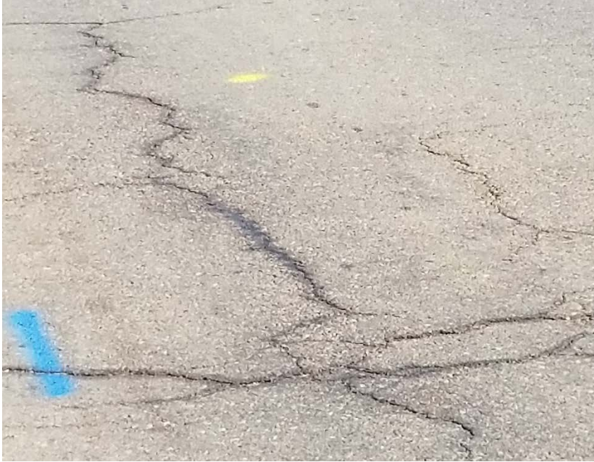
Liquid hydrocarbons emerging through cracked pavement on Tipple Parkway
