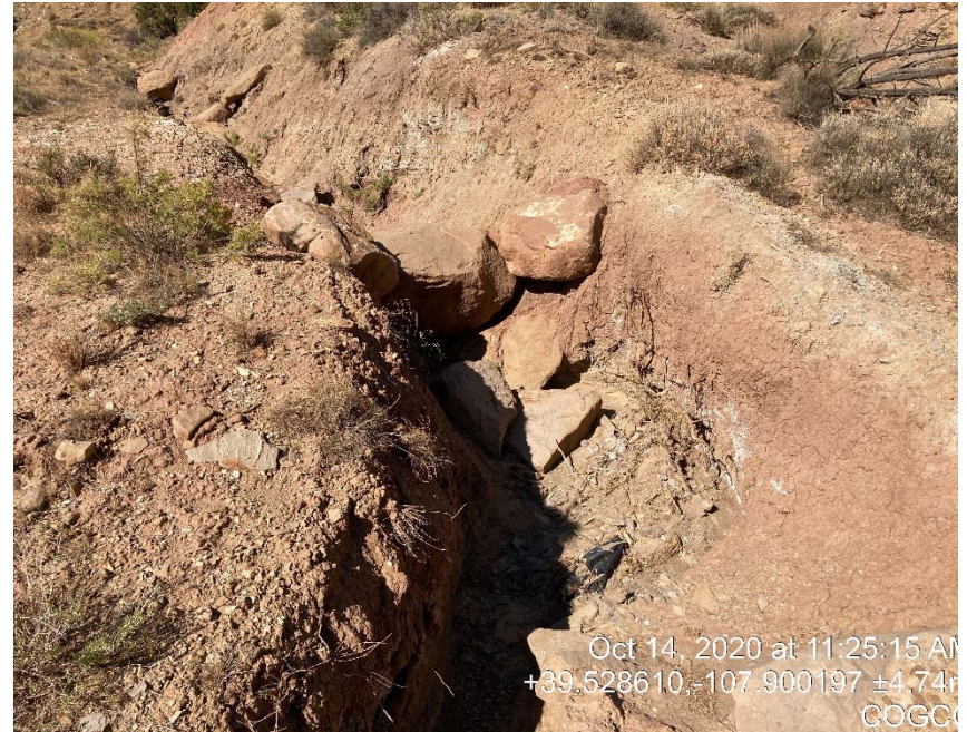
Erosion undercutting of BMP's
