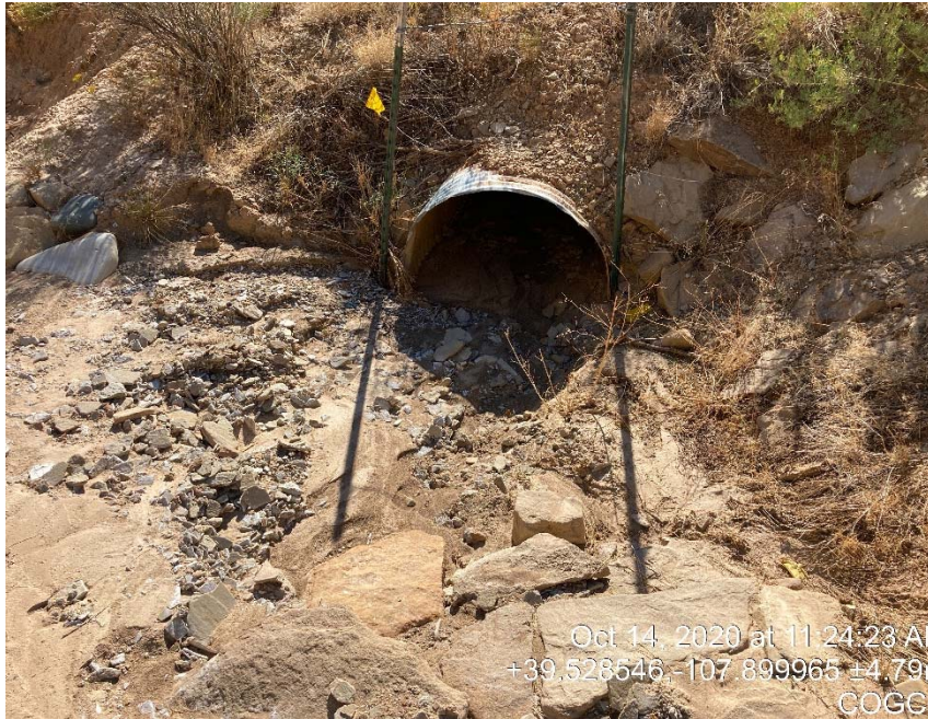
North side of road at entrance to location sediment going through culvert.
