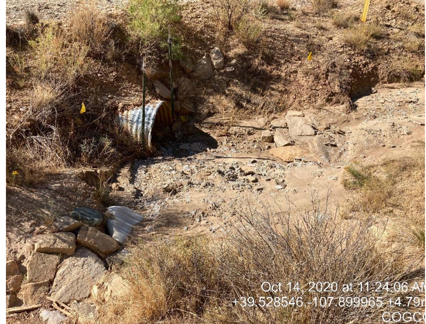
North side of road at entrance to location sediment going through culvert.
