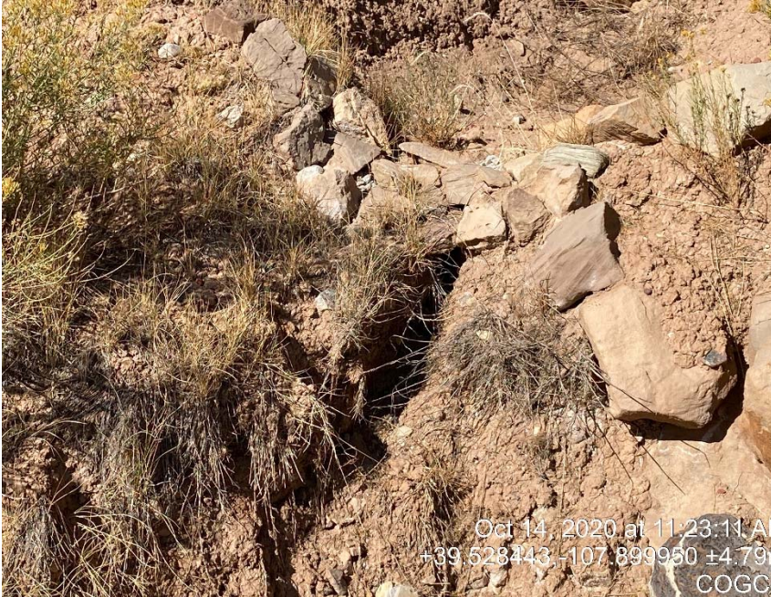
Erosion undercutting of BMP's
