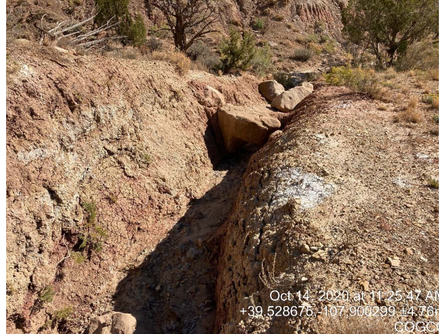
Erosion undercutting of BMP's
