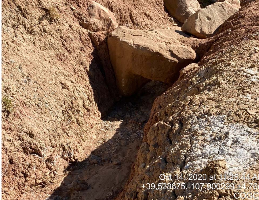
Erosion undercutting of BMP's
