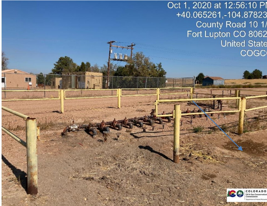
Pic 1 stained soil on manifold
