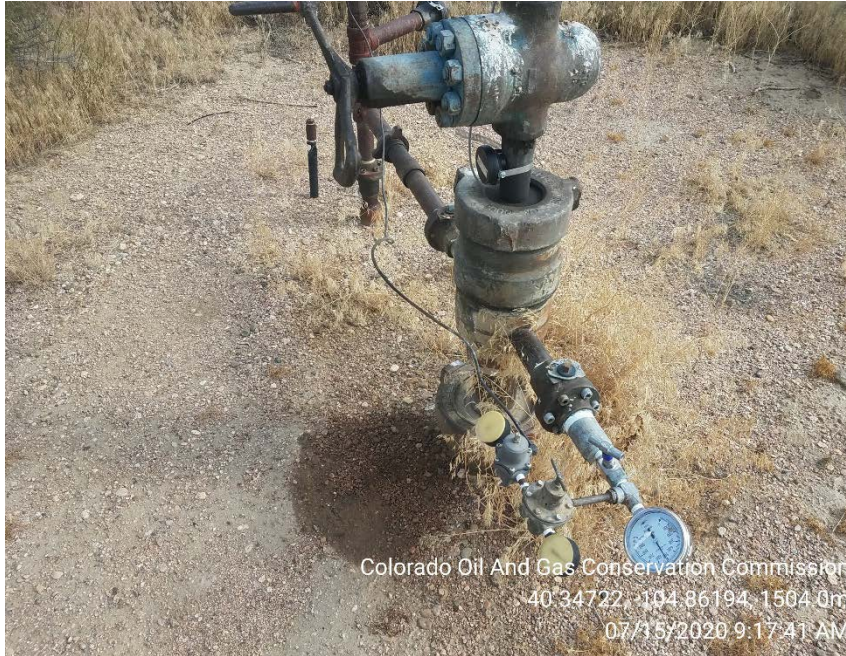
Master valve leak and stained soil on 7/15/2020
