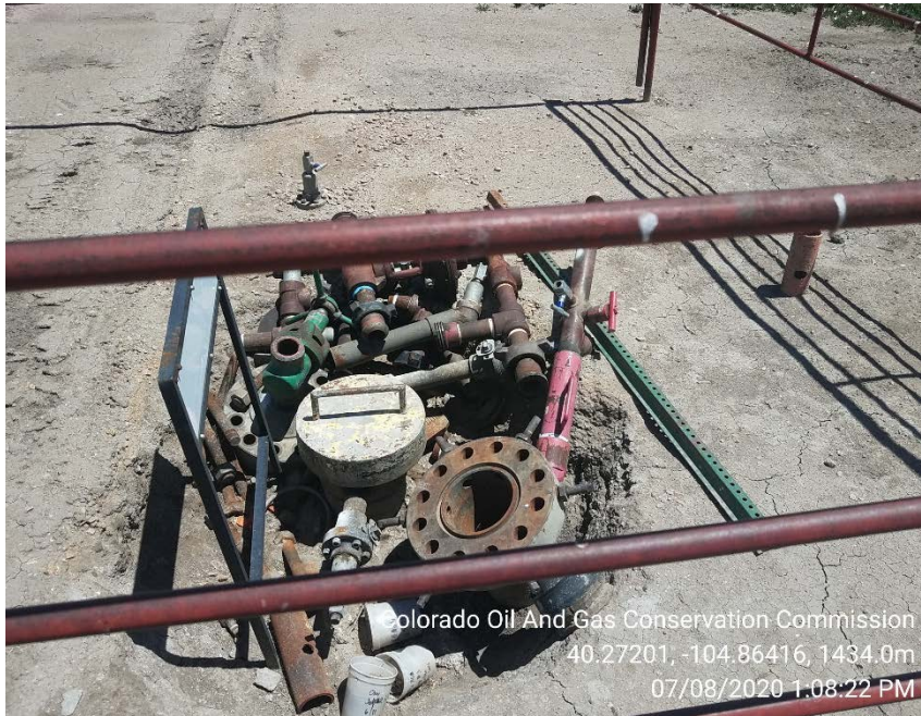
Unused equipment on 7/8/2020
