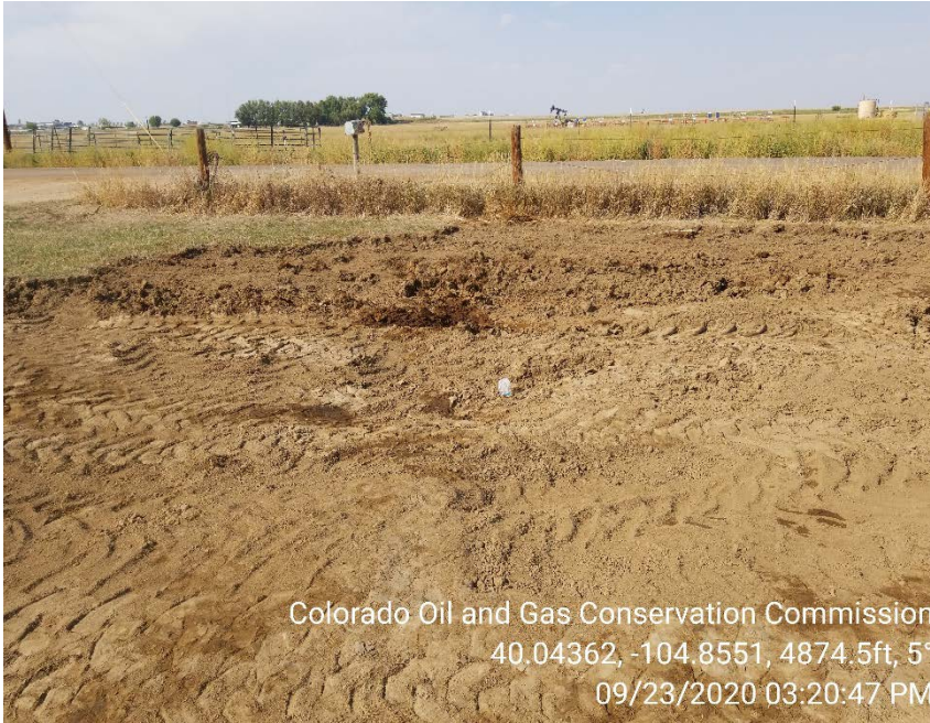
Photo 5 – Surface soil/vegetation removed from spill area. Pooled fluids observed in insp doc#689501090 have been removed
