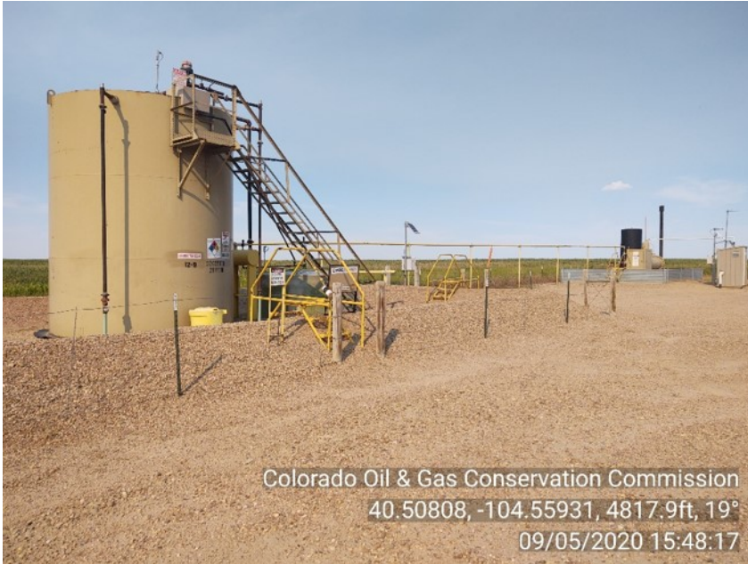
Photo #3 Erickson 24-4, 14-4 Battery site Active prior insp.
