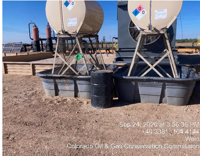
55 Gallon Drum needs secondary containment
