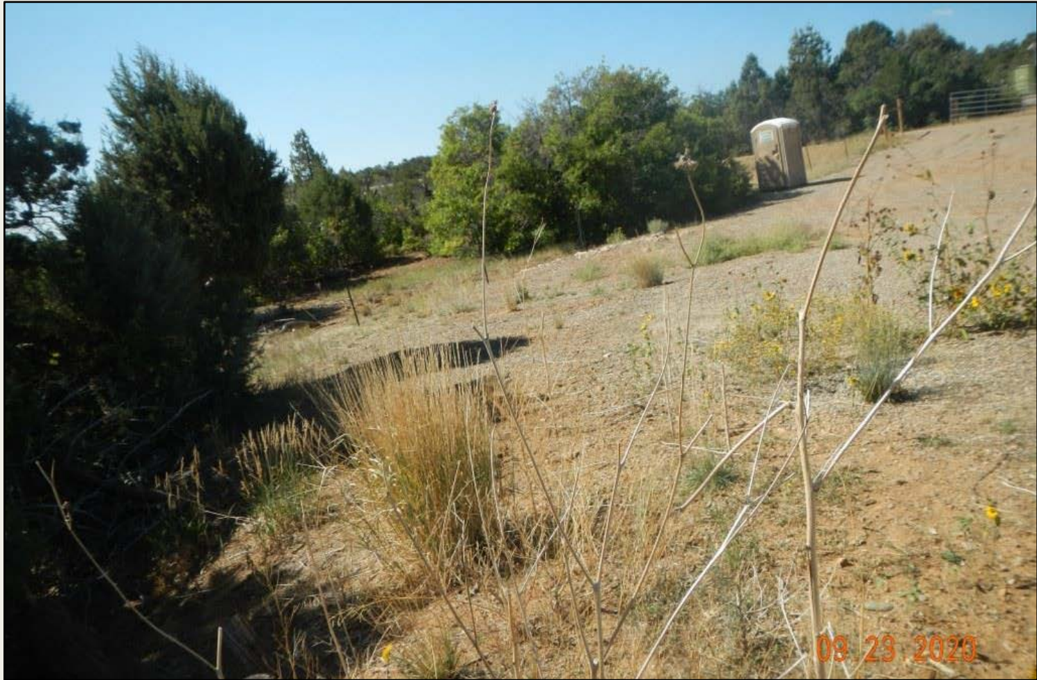
Photo 2. View of the southern fill slope from the southeastern corner facing westward.
