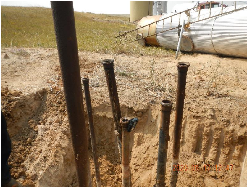
Photo 1: View of Trimble GPS unit on center flow line riser at heater treater site.
