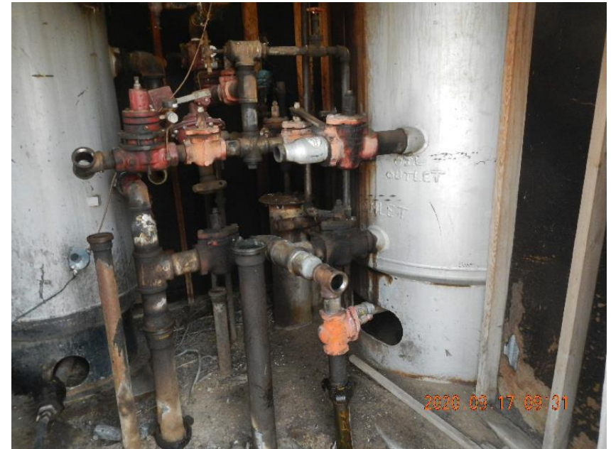
Photo 2: Disconnected lines for treaters inside heater treater shed.
