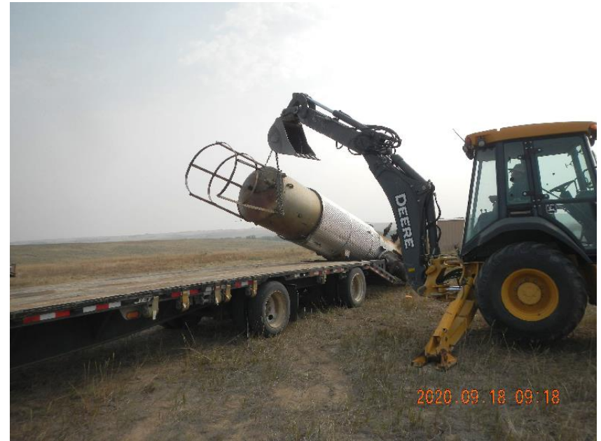
Photo 14: Loading heater treater for haul off.
