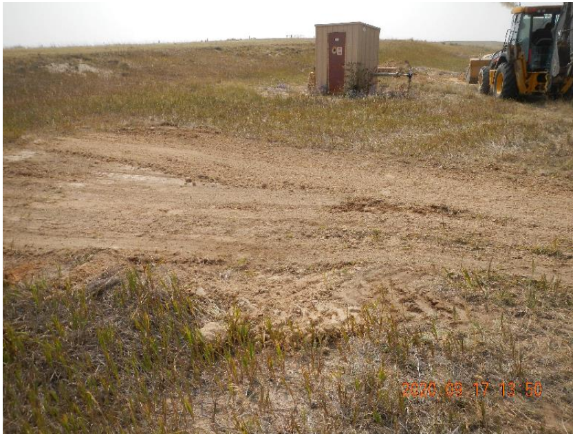
Photo 11: Backfilled and dressed excavation site on E side of meter run shed.
