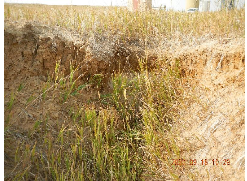
Photo 20: View from inside erosion gully looking at top of erosion.
