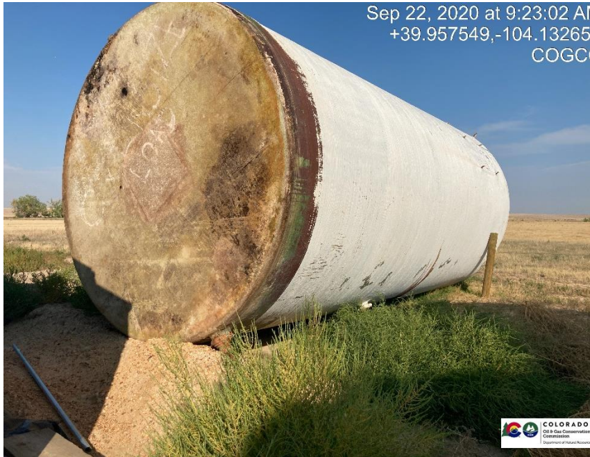
Pic 9 weeds / storage of equipment
