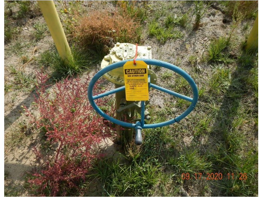
Tagged out valve north of release point.
