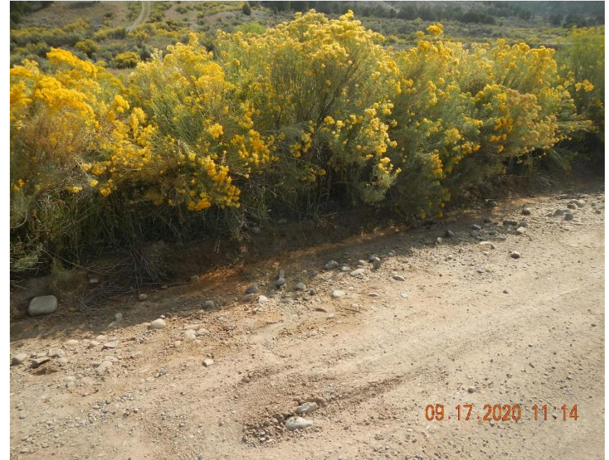
Wet and stained soil observed in roadside ditch.
