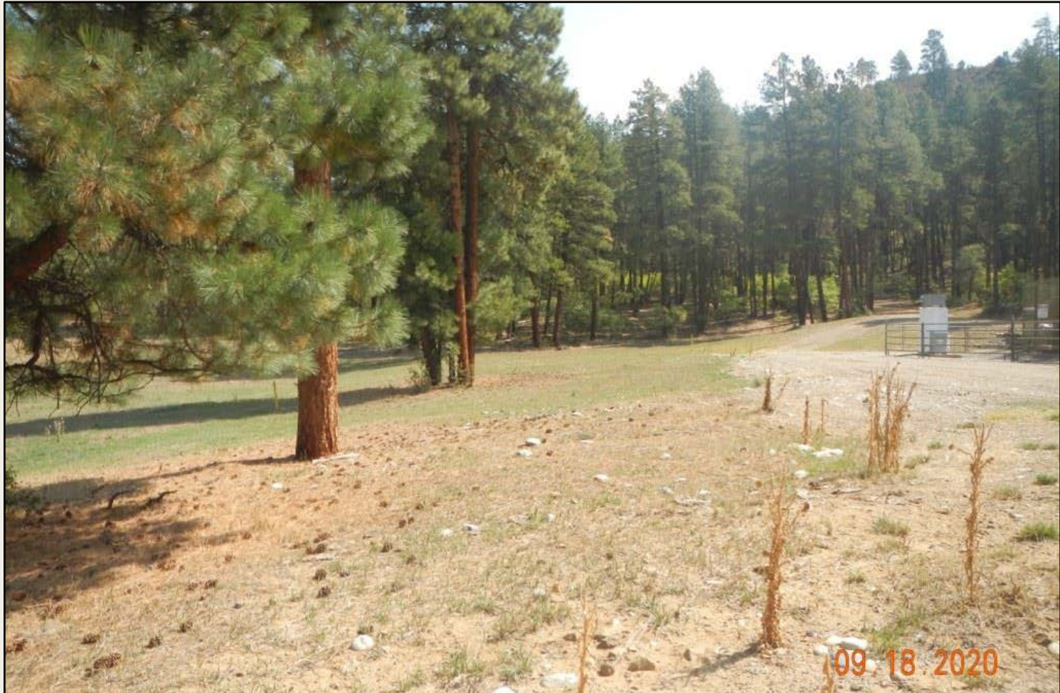
Photo 2. View of the northern fill slope from the northwestern corner facing eastward. Revegetation is progressing with grasses such as western wheatgrass and sand dropseed, largely in a grazed condition. Musk thistles appear to be herbicide treated in a post-flowering condition.
