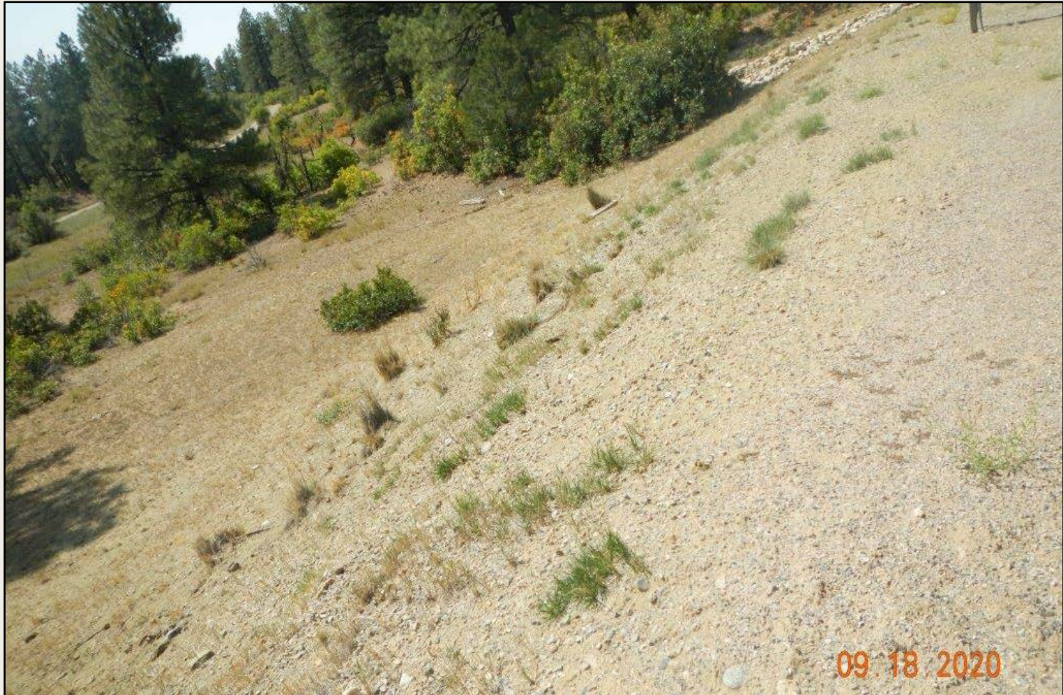
Photo 3. View of the southern fill slope from the southeastern corner facing eastward.
