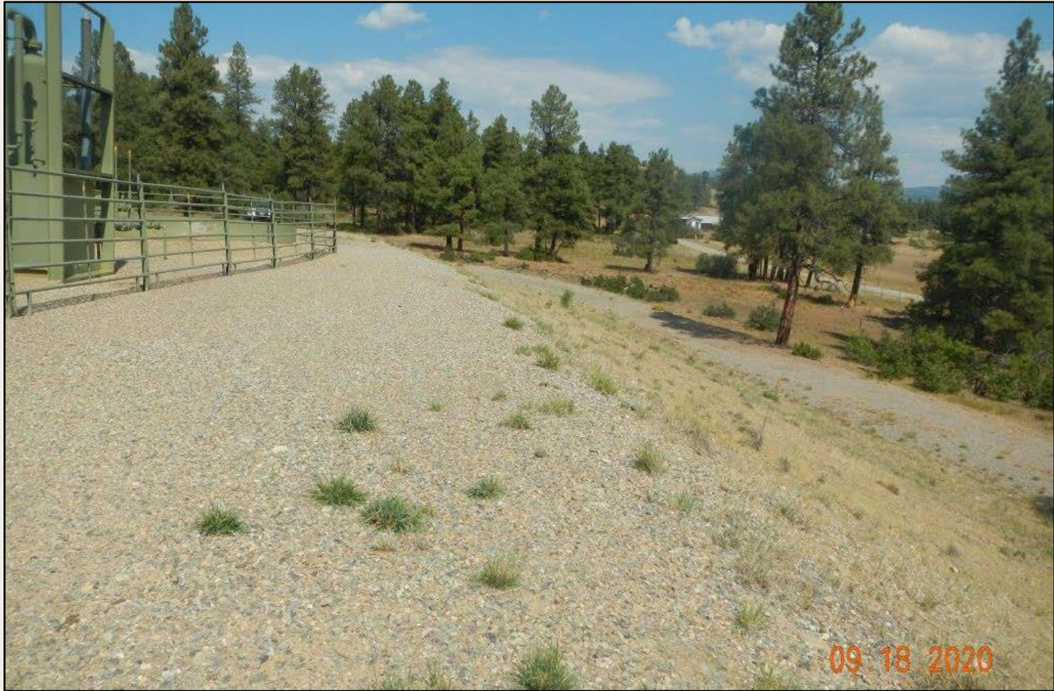
Photo 2. View of the eastern fill slope from the southeastern corner facing northward. Revegetation is progressing with grasses such as western wheatgrass and sand dropseed, largely in a grazed condition.
