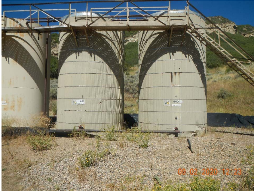
Photo 6. Example of tank labels tearing/fading. Weeds.
