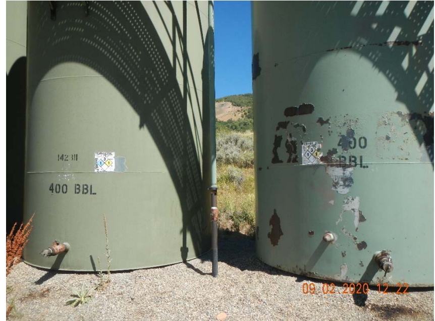
Photo 5. Example of tank labels tearing/fading.
