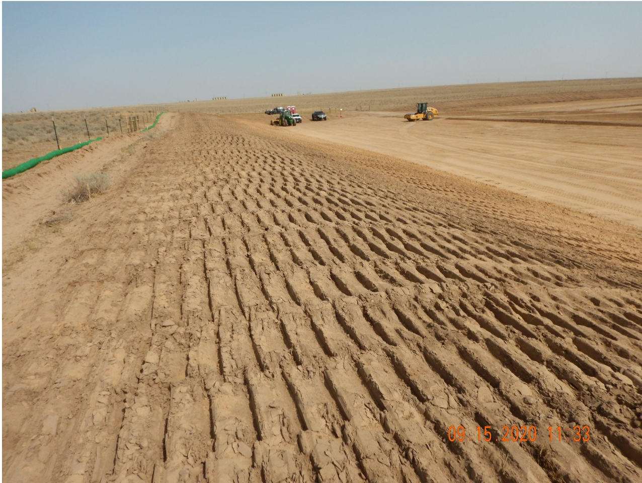
Photo 6. Photo taken from the southwestern location, facing North. Photo illustrates the cut slope has been temporarily stabilized with equipment tracking.
