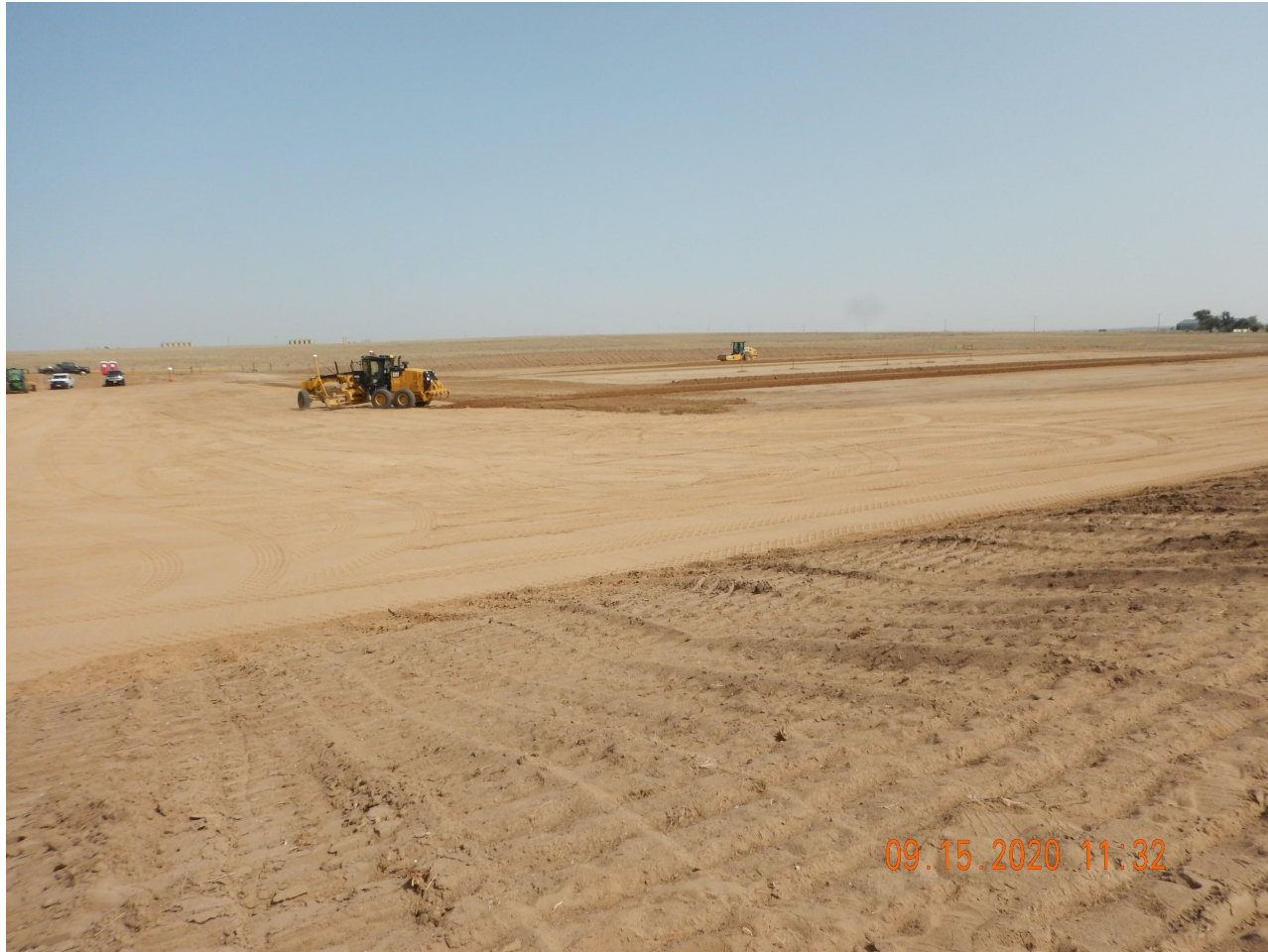
Photo 7. Photo taken from the southwestern location, facing Northeast. Photo illustrates Operator is in process of added roadbase to the location.
