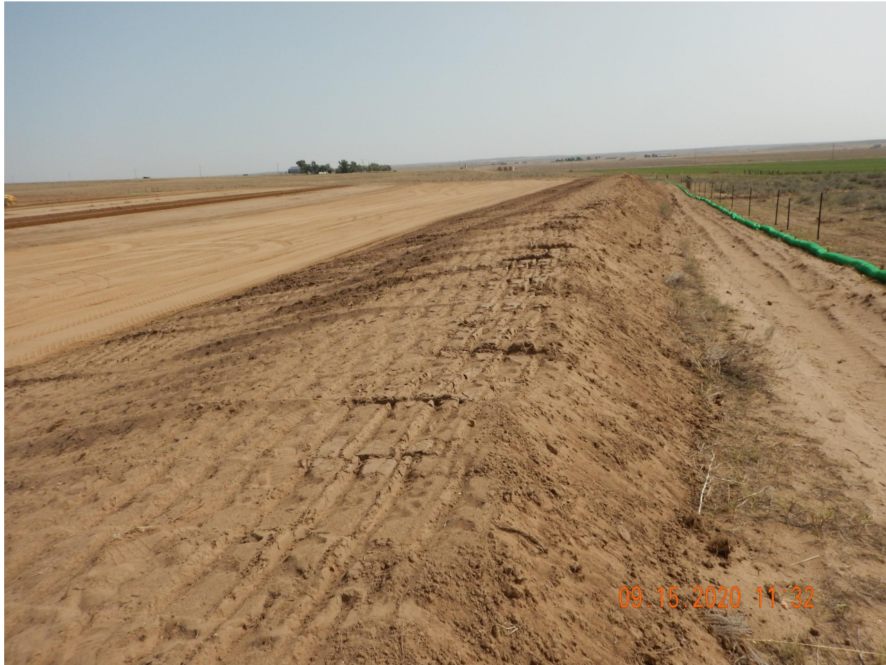
Photo 6. Photo taken from the southwestern location, facing East. Photo illustrates the second topsoil stockpile which has been temporarily stabilized with equipment tracking.
