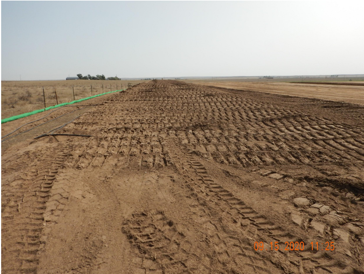
Photo 2. Photo taken from the northwestern location, facing East. Photo illustrates one of two topsoil stockpiles. Most of the stockpile has been temporarily stabilized with equipment tracking and planned operations will be performed for long-term stabilization.
