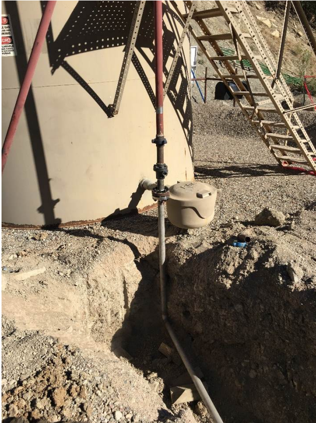
New 2" stainless steel dump line riser at tank battery
