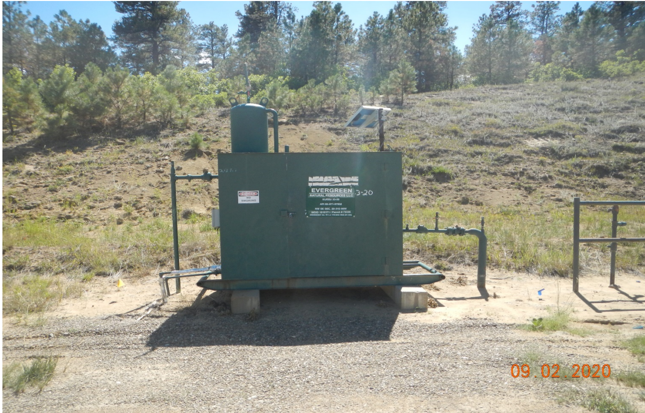
Photo 2. Well sign posted at meter shed.
