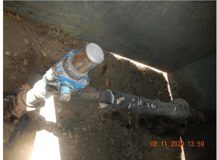
Photo 2. Photo of wellhead inside housing.
