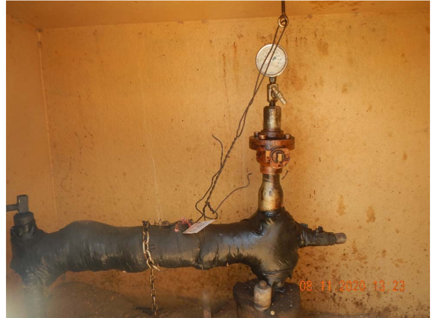
Photo 2. Wellhead inside housing.
