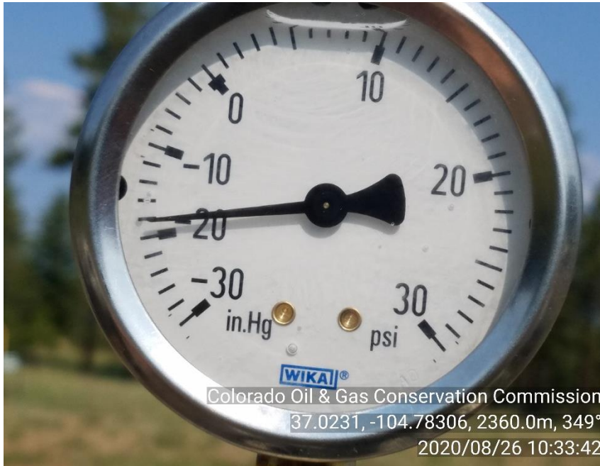
PHOTO 3: INJECTION PRESSURE GAUGE.
