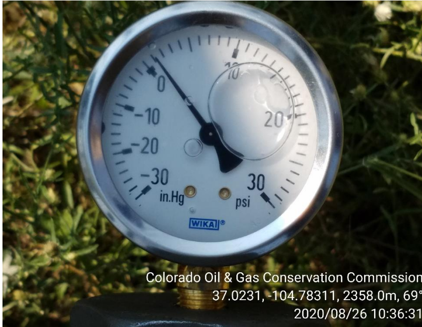
PHOTO 5: BRADENHEAD PRESSURE GAUGE.
