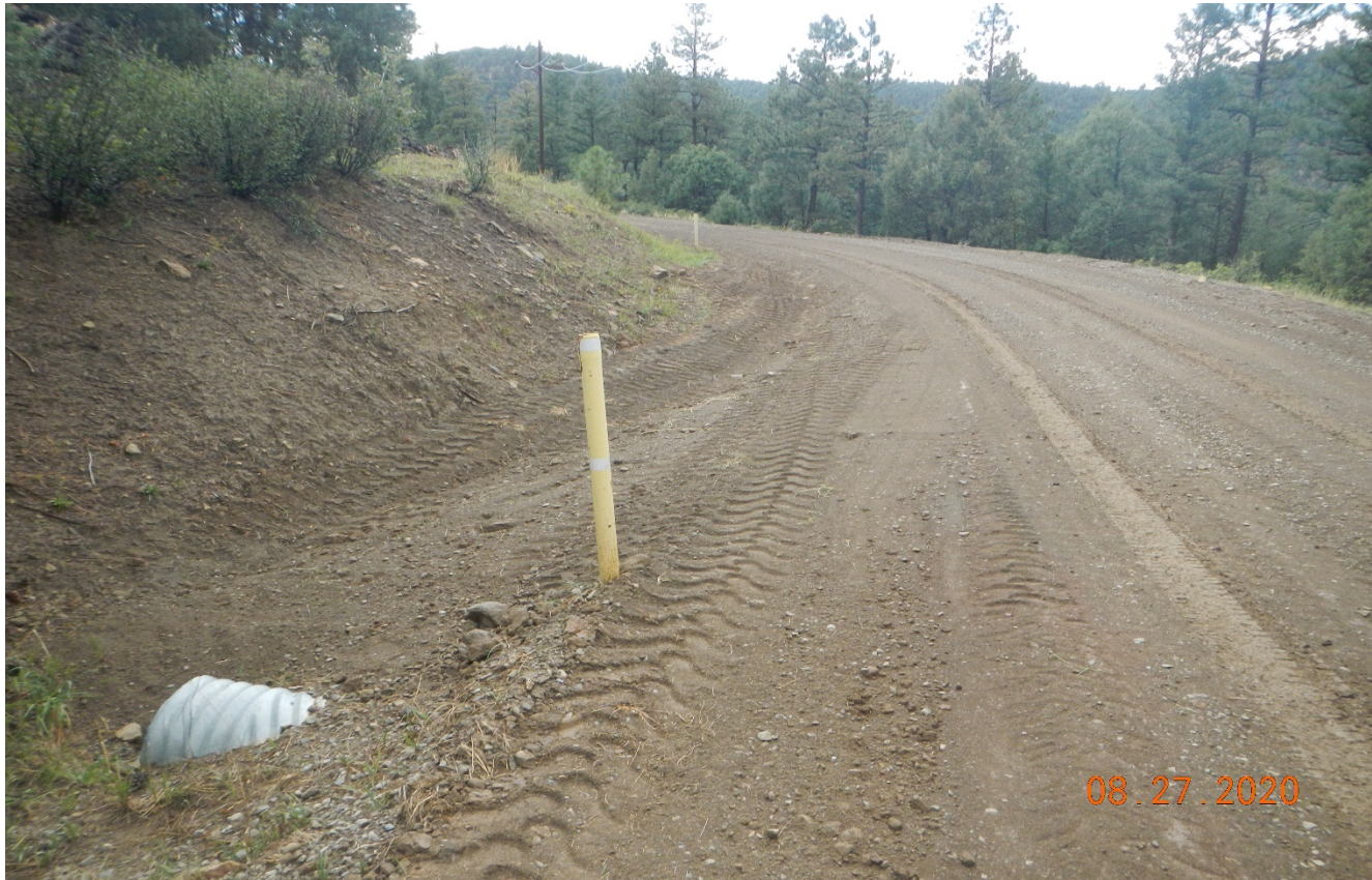
Photo 1. The road has been regraded near the location and the culvert is maintained.
