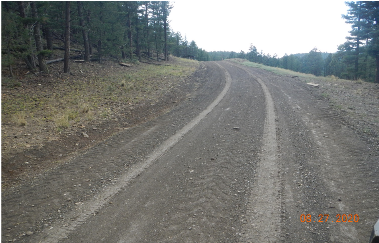
Photo 2. Facing west near the location. The erosion has been repaired and road regraded. BMP's may be needed along the road to dissipate stormwater flow.
