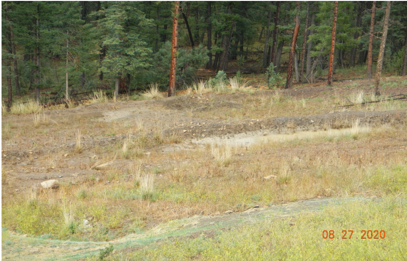
Photo 4. The berms along the bottom of the fill slope have been repaired.
