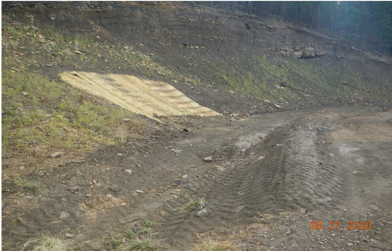
Photo 3. There is straw blanket installed along a portion of the cut slope.
