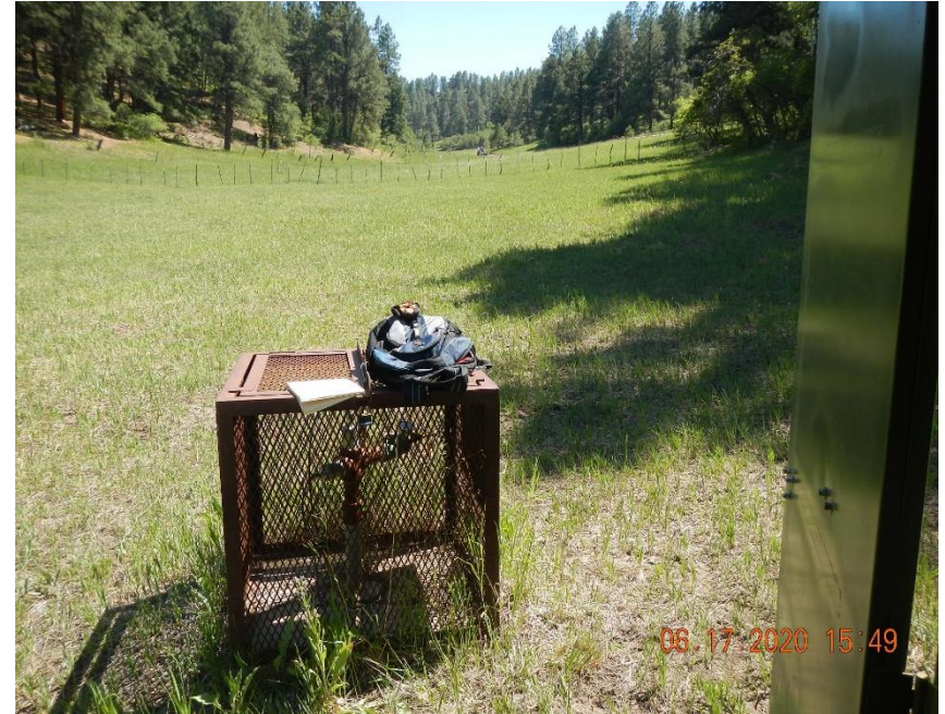
Monitor Well 35-7-8 #2 well head and protective metal cage enclosure.
