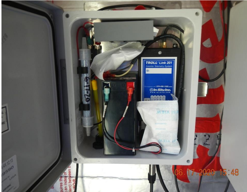
Fresh desiccants installed in Troll Link 201 equipment enclosure.
