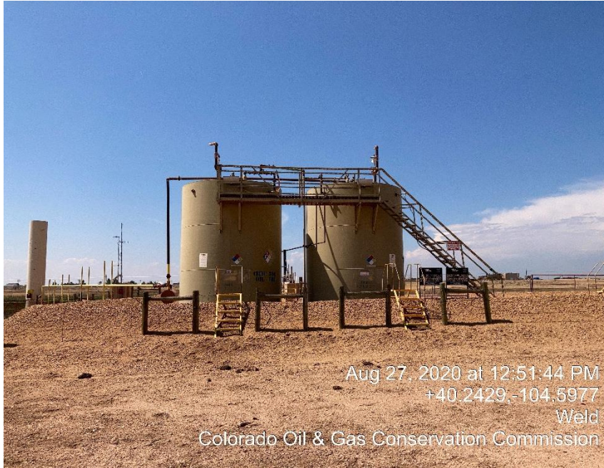
Photo #3 Tank Battery
