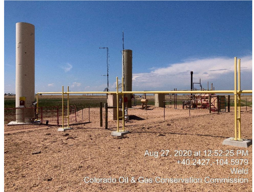
Photo #4 Separator, ECD's & Meter Runs
