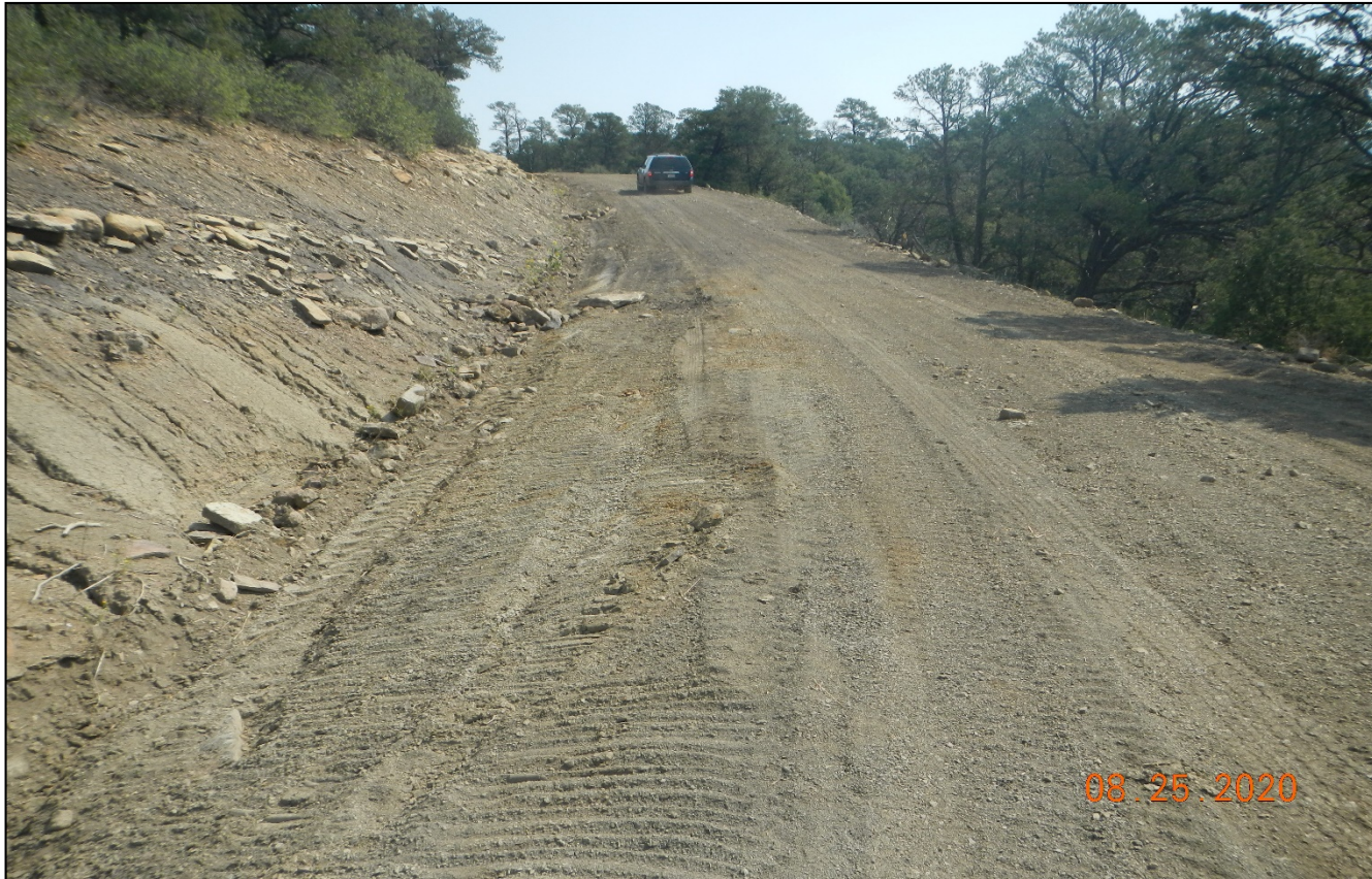
Photo 6. Facing southeast along the road ascending the hill side. The road was reggraded along a portion of the road. Additional rock check dams are needed along the side of the road to dissipate stormwater flow and prevent erosion.
