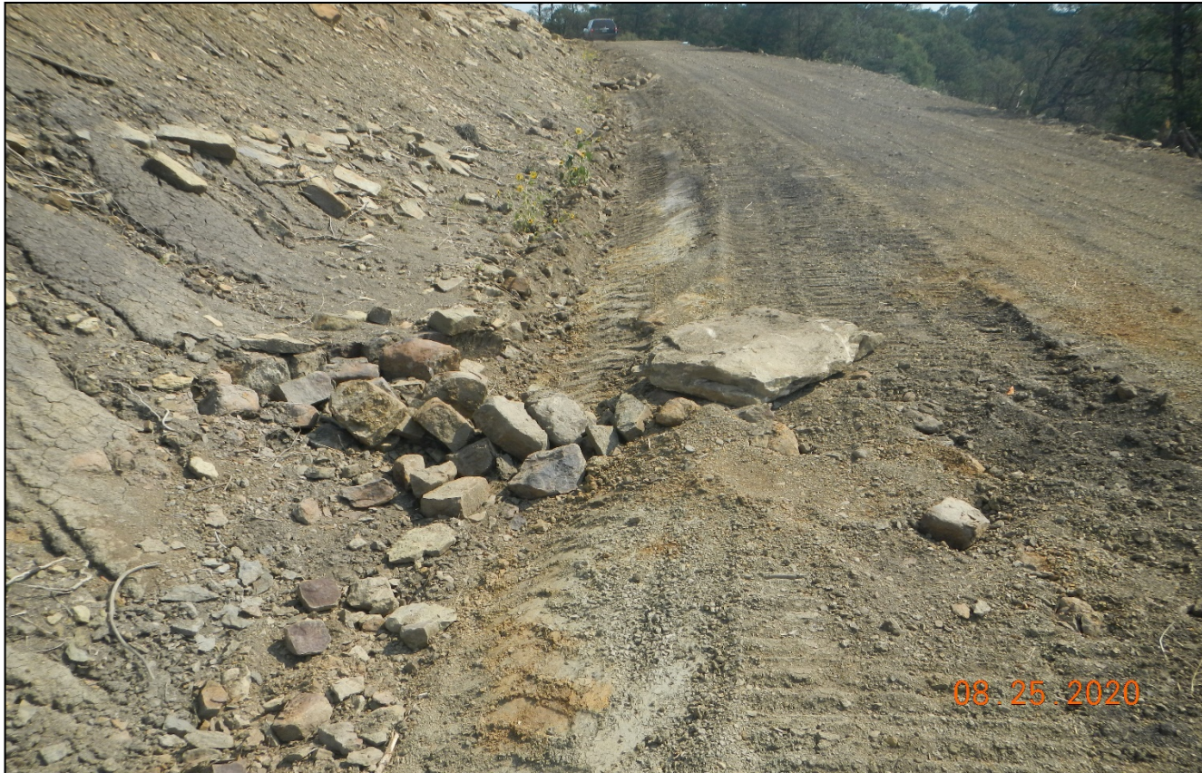
Photo 7. The rock check dams are not properly installed along the road side. Additional rock is needed and the check dams need to extend from side to side with the low point at the center of the check dam.
