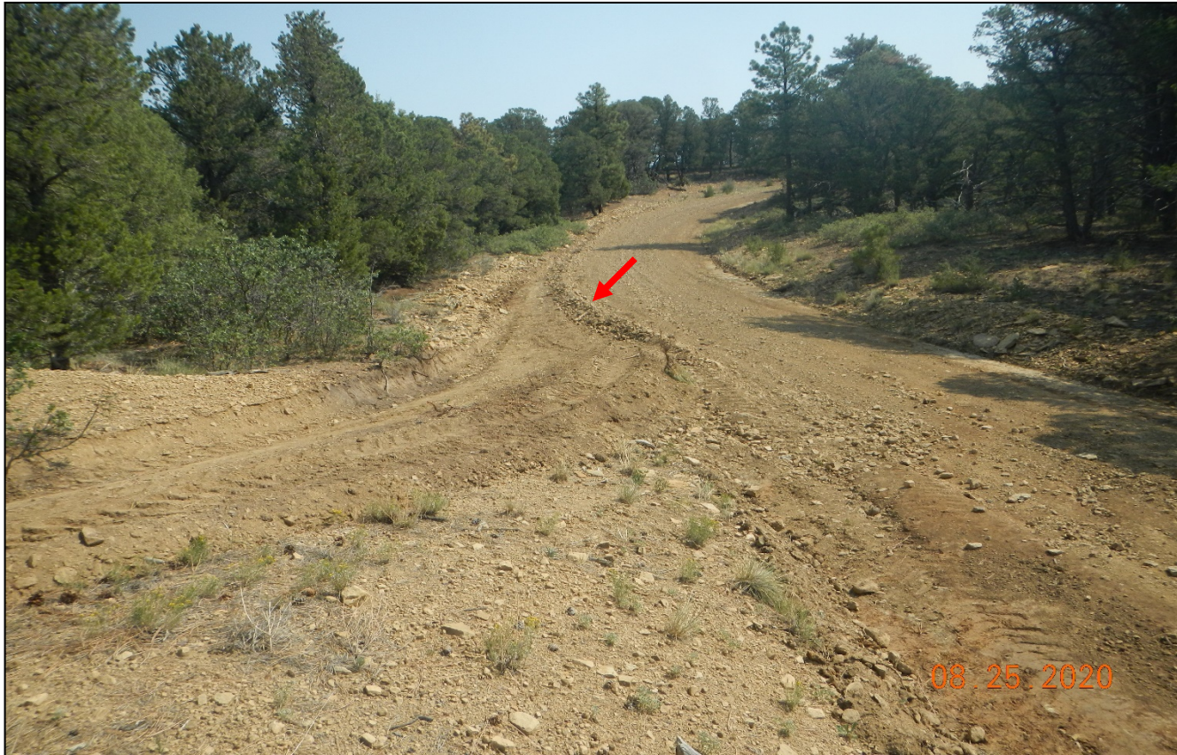
Photo 10. Facing east along the road. This area of the road was regraded however, a berm was left on the road which will interfere with stormwater flow.
