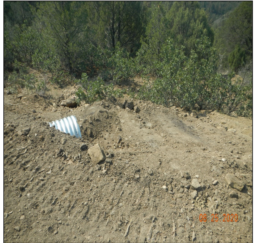
Photo 5. There is no culvert outlet protection installed to prevent erosion.
