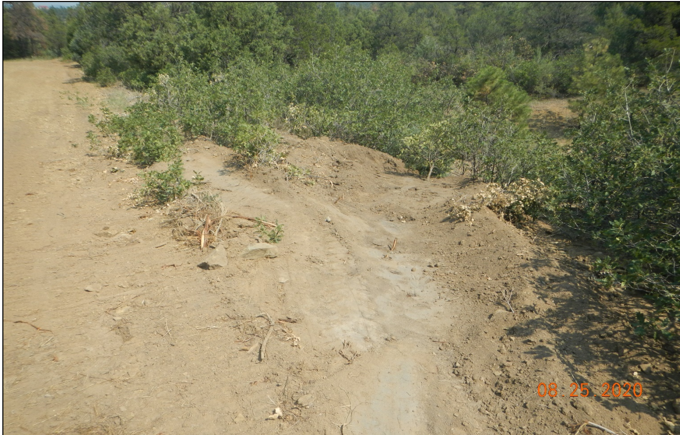
Photo 2. This runoff ditch was not properly installed. The disturbance along the side of the road will need to be seeded and stabilized.
