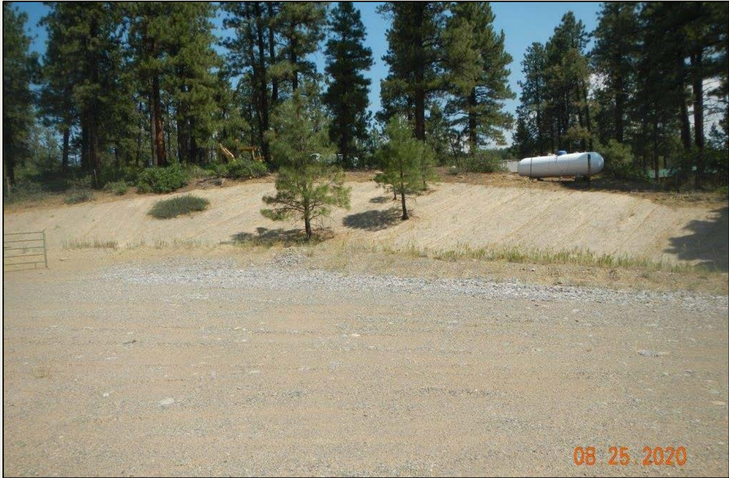
Photo 2. View of the northern cut-slope. Erosion control blanket installed along the slope.
