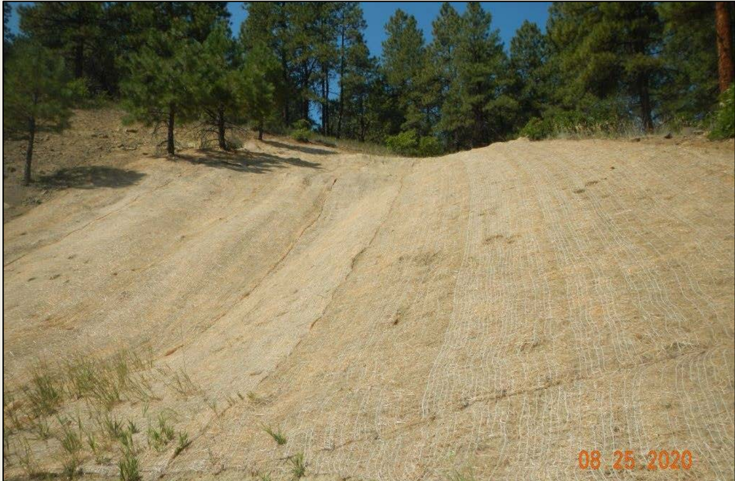
Photo 3. View of erosion control blanket installed in the southwestern project area. Small smooth brome plants observed near the toe of the slope.
