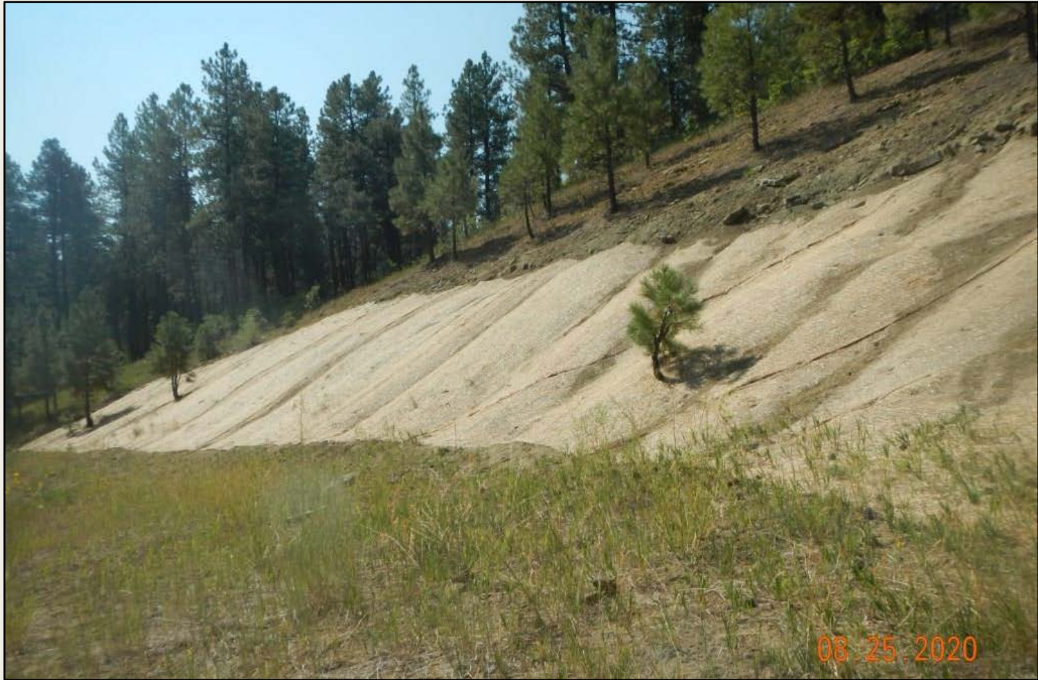
Photo 2. View of erosion control blankets installed on the southern cut-slope. Blankets appear to be properly installed.
