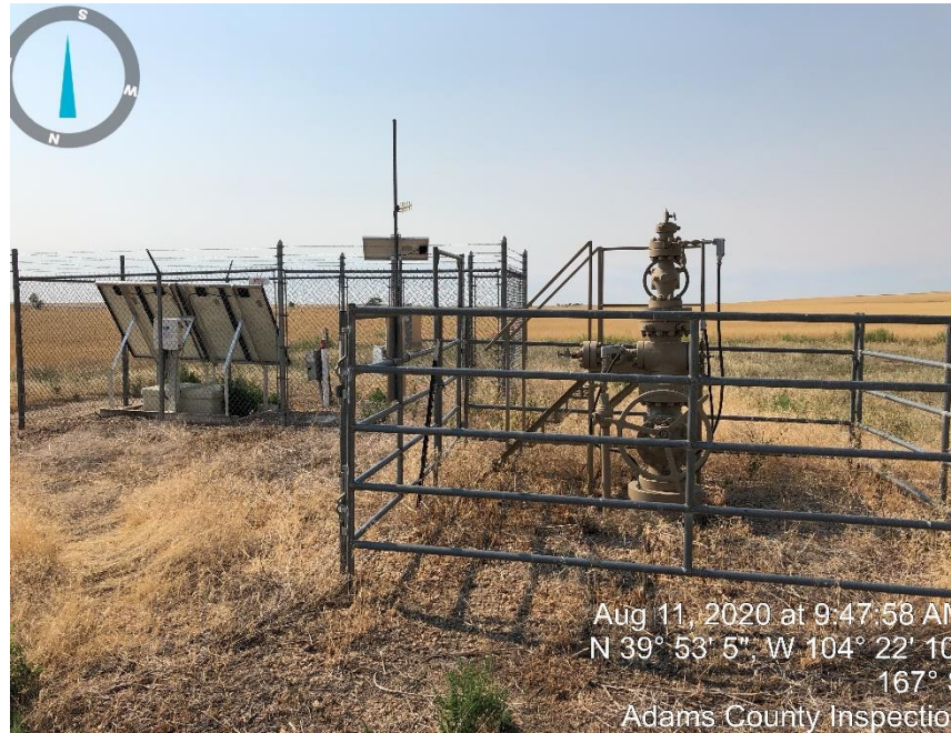
Photo #1 Well head & RTU.
