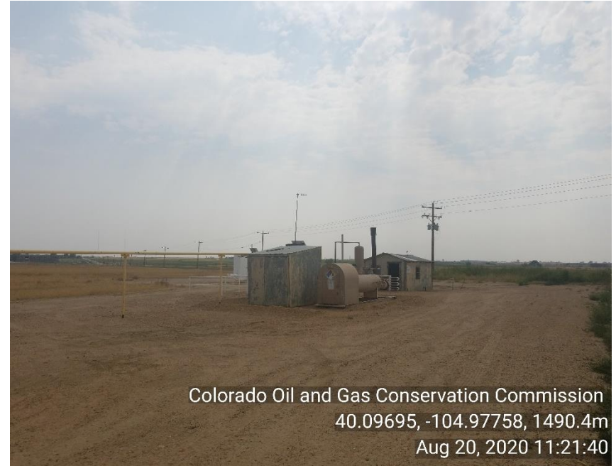
Photo 4 Separator, ECD meter house and Electric compressor.
