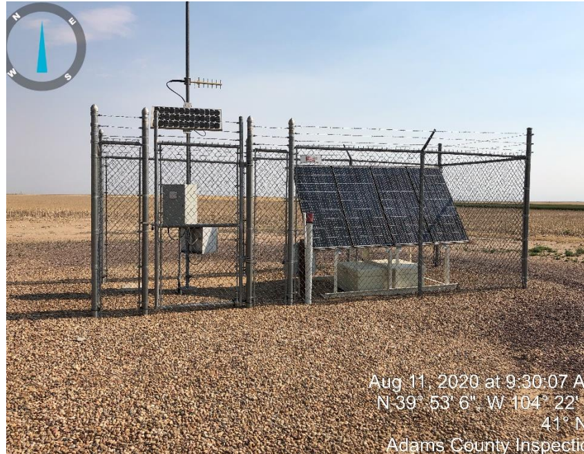
Photo #3 ancillary equipment.
