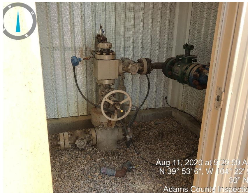
Photo #2 well head
