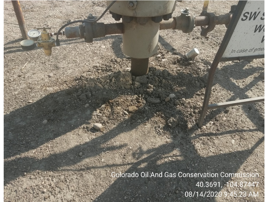
Stained soil on 8/14/2020
