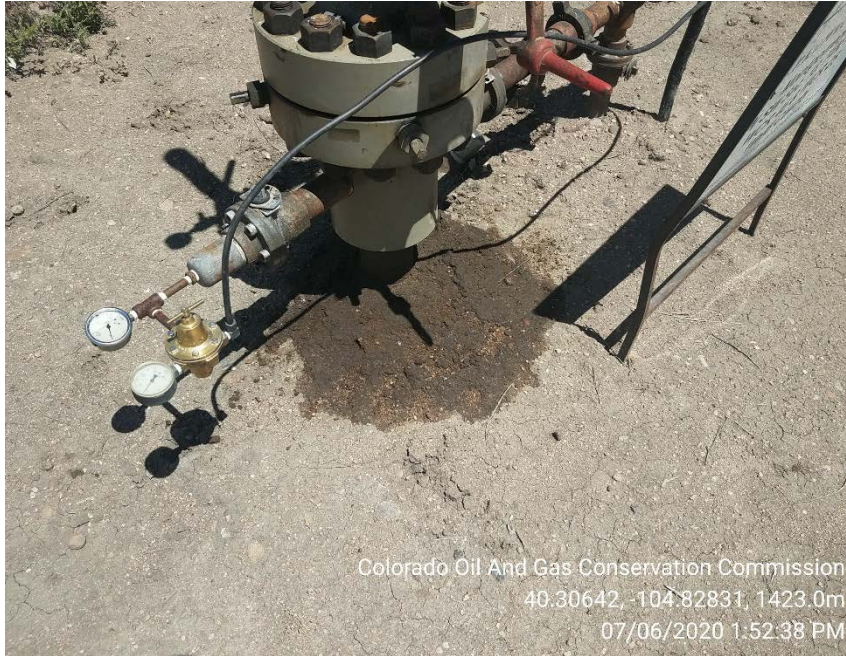
Stained soil on 7/6/2020
