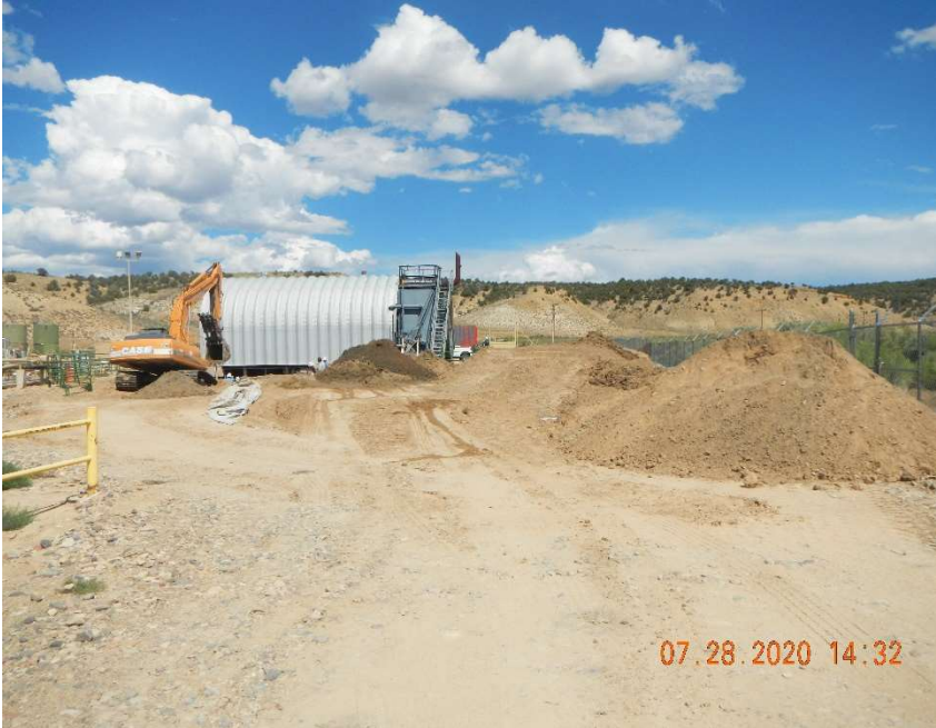
Spill/Release location, photo taken from Co Rd 20.
