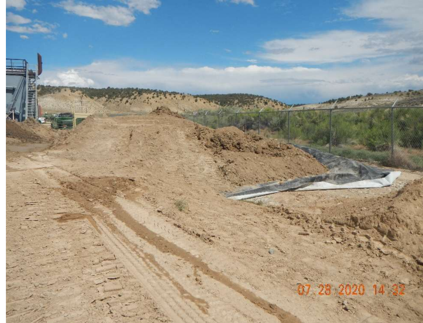
Stockpiled material from the excavation, note the fluids and areas where the impacted material is not properly stored on the liner material.
