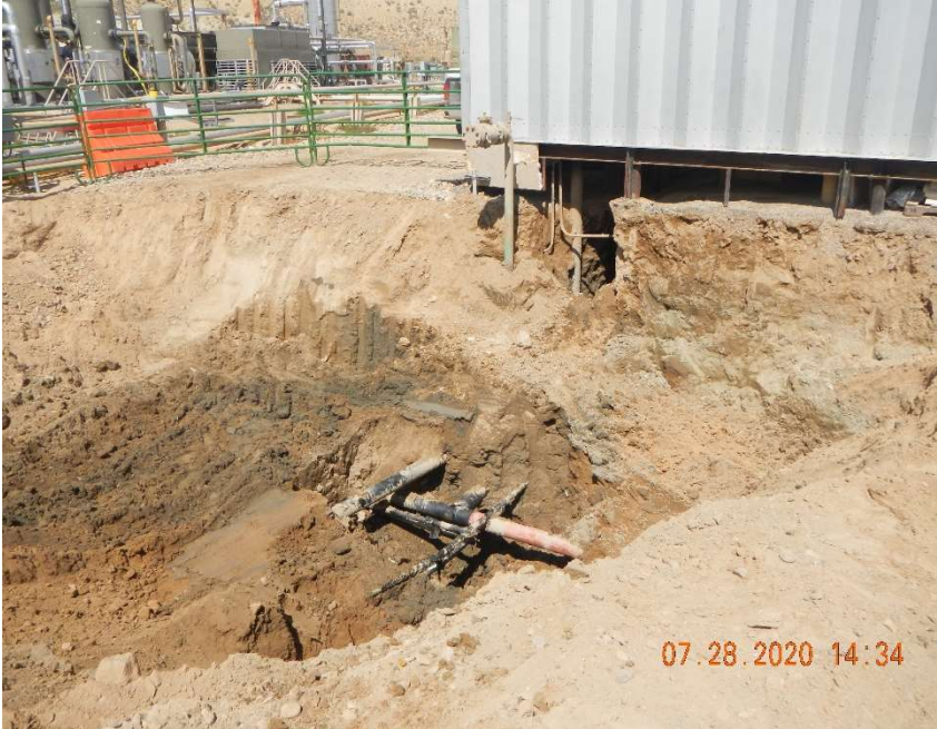
Excavation looking east, note the stained soils on the sidewalls and bottom of the excavation.
