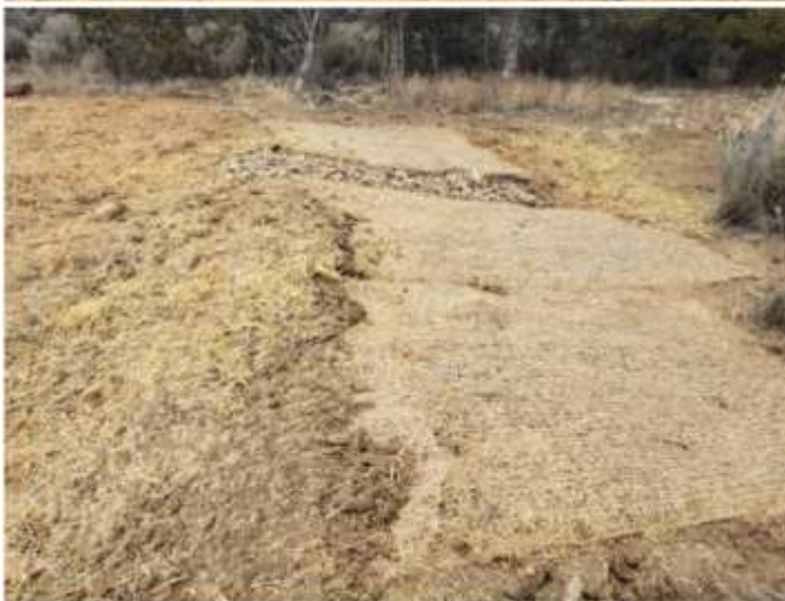
During equipment removal work performed by Red Cedar on their items left on pad additional disturbance was created so those areas were seeded and mulched for stabilization as well. Additional
