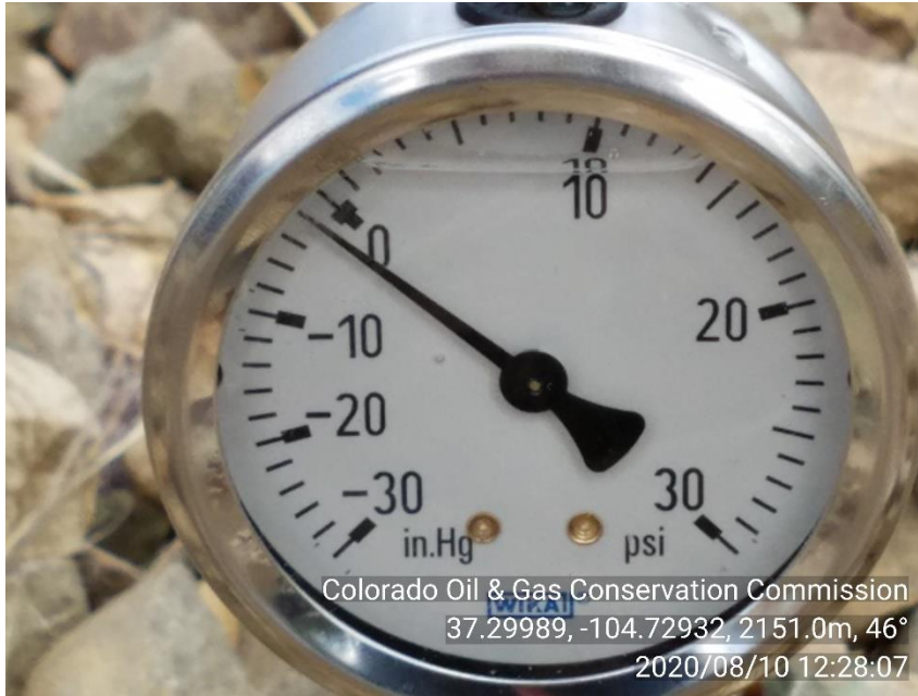
PHOTO 5: BRADEN HEAD PRESSURE GAUGE
