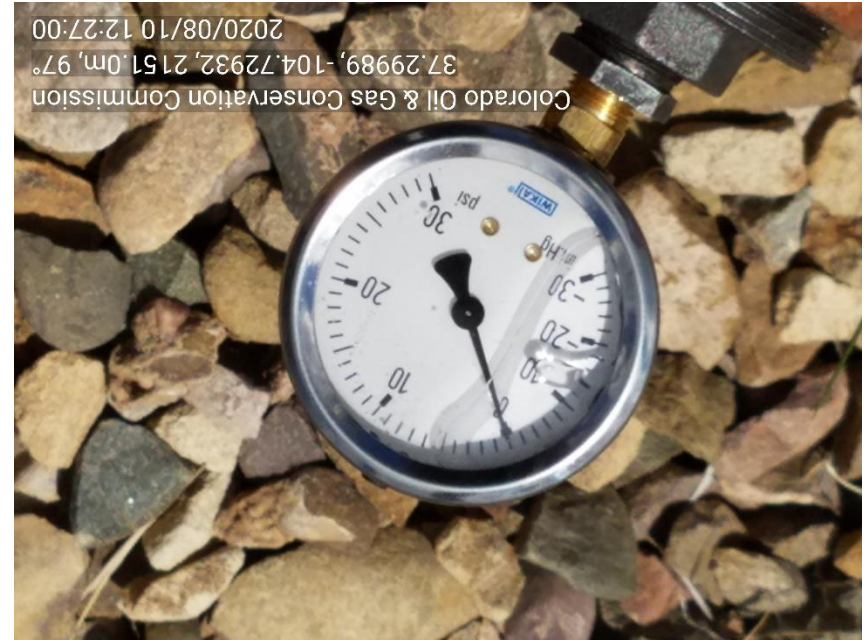
PHOTO 4: PRESSURE GAUGE FOR ANNULUS BETWEEN TUBING AND CASING.
