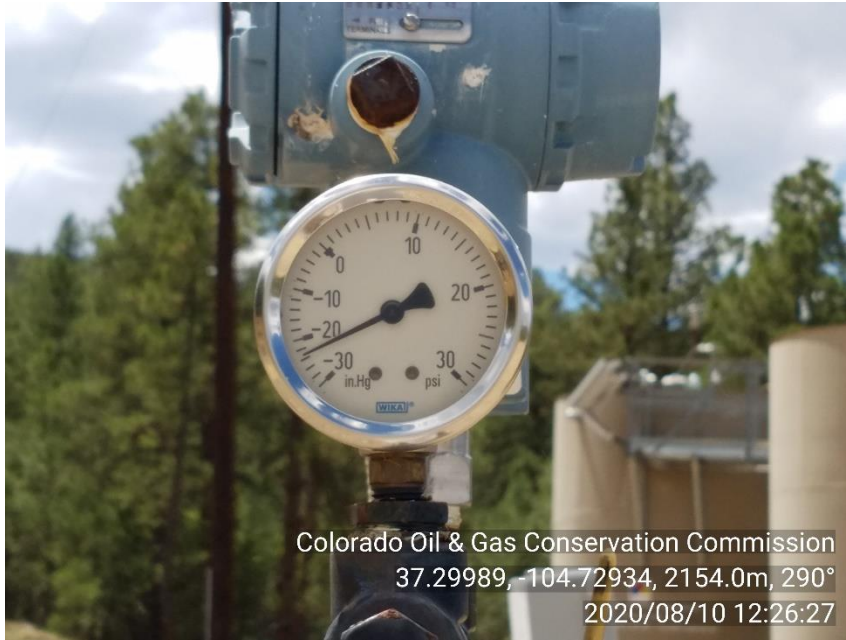
PHOTO 3: INJECTION PRESSURE GAUGE
